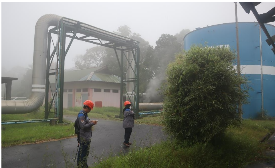
Gambar 8. Area Cooling Tower I
